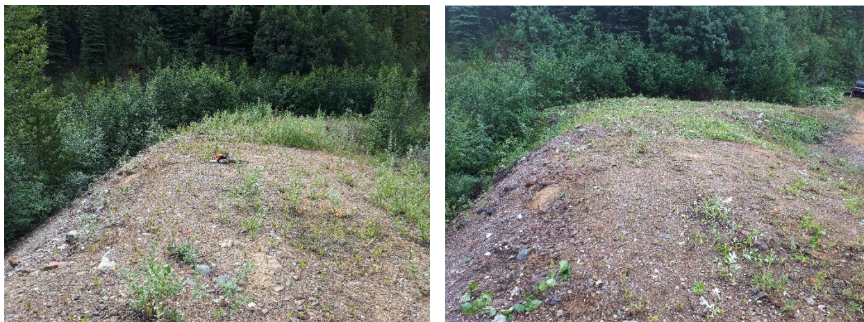
Figure 14. Before (L) and After (R) of brushing work conducted on a Tailings Storage Facility for proper maintenance.
